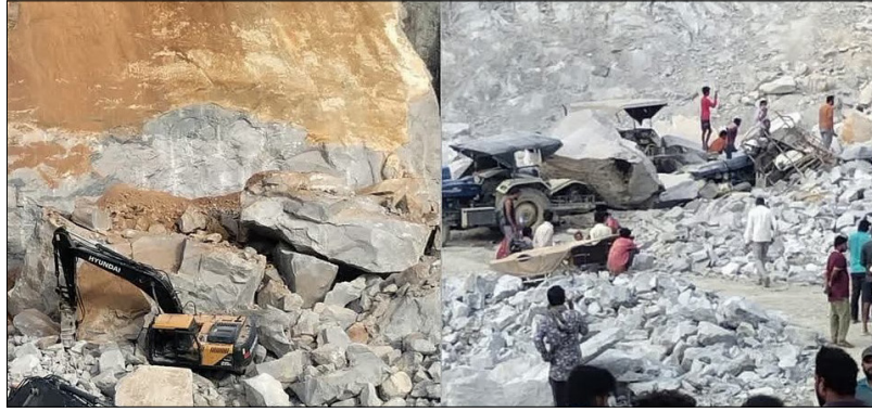
During the process, a large rock allegedly dislodged from a height of around 40 feet and came crashing down into the quarry pit, trapping workers underneath.
